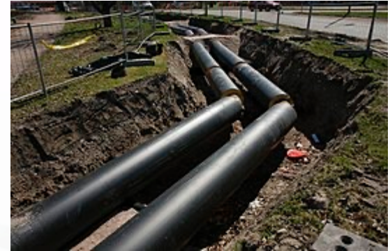
Piping cost is a large part of the investment.
